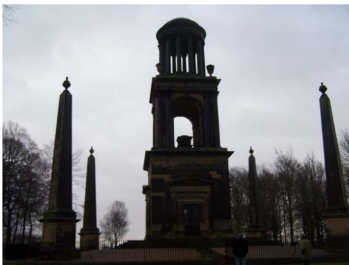
The Rockingham Mausoleum. Note the as yet little-soiled replacement stonework, as well as the cleaner sections beneath cornices, illustrating the limit of effectiveness of drips. Also the grey chemical cleaning test panels to the lower right-hand corner
